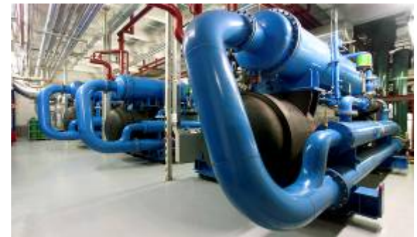
30 MW cooling capacity
